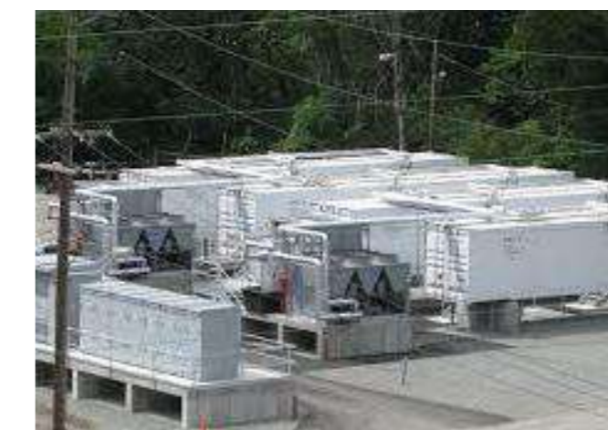
Long duration utility scale batteries
