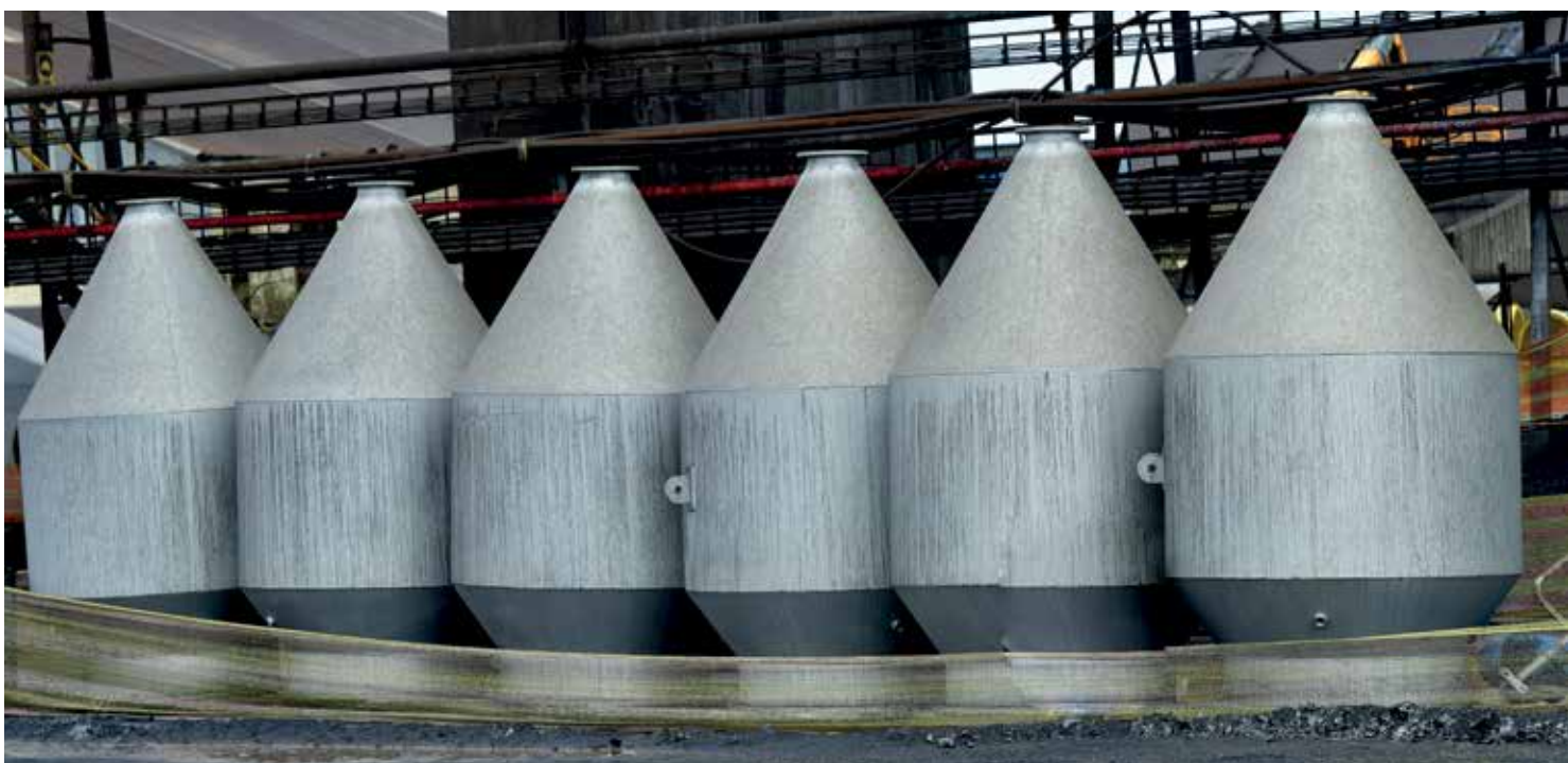
Components of the Off Gas Scrubber Unit
