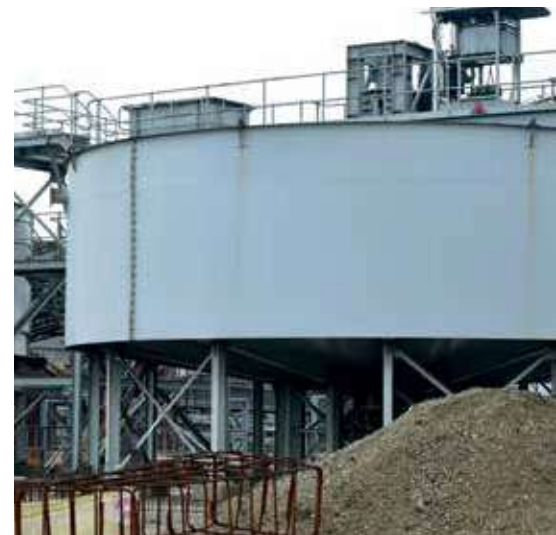
Thickener for the Off Gas Scrubber Unit
