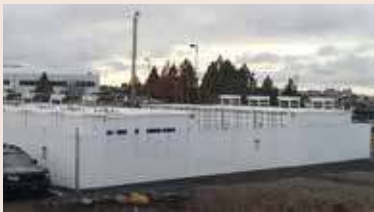
VRFB installation example – the UET system with Avista in Pullman, WA, USA – commissioned in 2015
