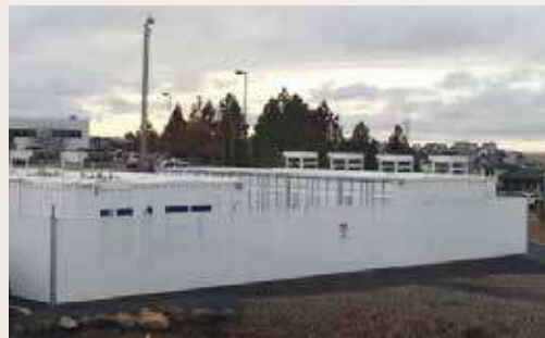
Operational 4MWh vanadium redox flow battery
