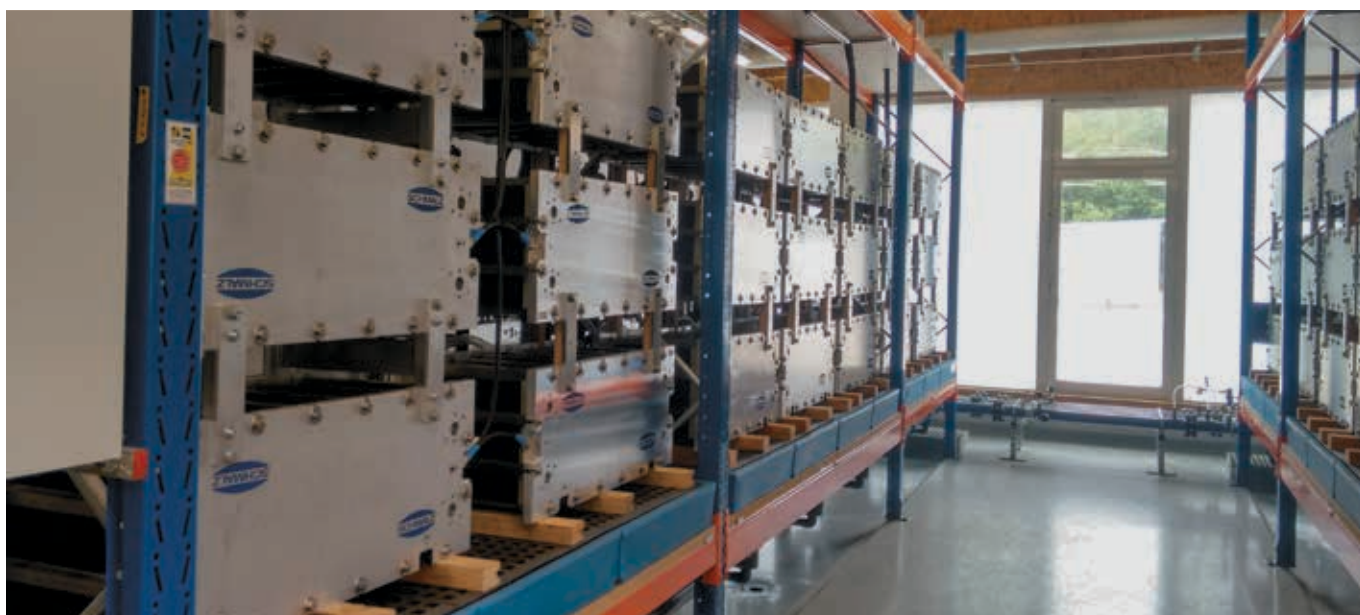
Cell stacks at the Fraunhofer ICT VRFB, Karlsruhe, Germany
